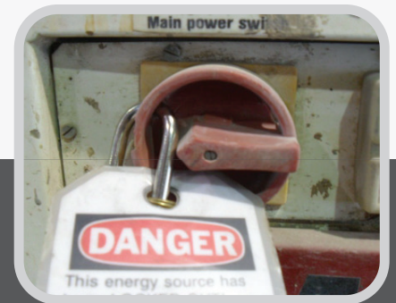
LOCKED OUT SWITCH
